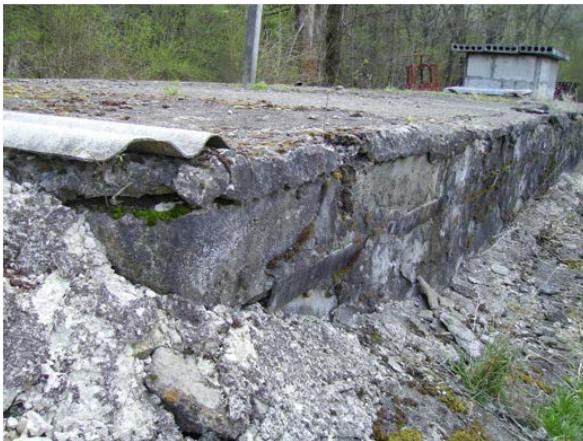
Fig. 7 Condition of the facility (Site Report, p.88).
