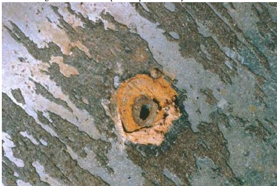
Figure 36: Microbial corrosion pit [Linhart P, 2006].
