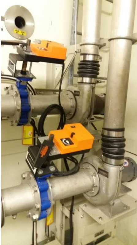
Figure 3-5. Aerosol sampling at B2: the activity monitoring system. Shows pumps in primary loops and flow regulating valves. The system at B1 has a similar design.
