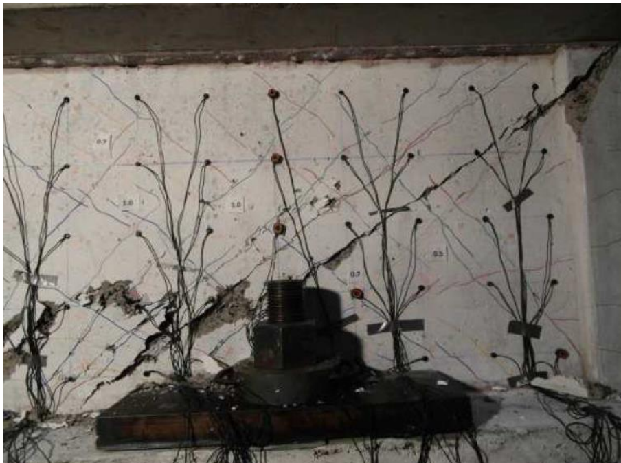
Figure 2-41 Picture of wall specimen ASR A1 (specimen with ASR reactive concrete) at failure [7].
