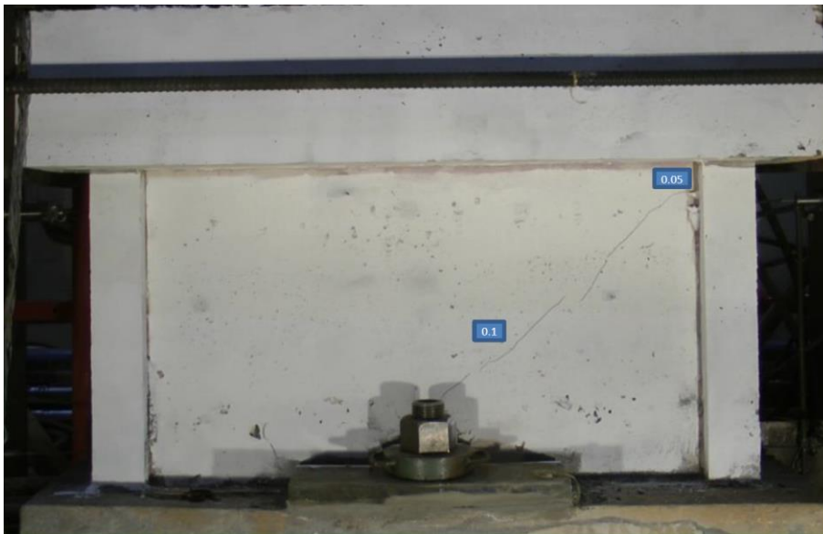
Figure 2-26 First crack at a load of 780 kN and a displacement of 1.4 mm of Reg B shear wall [15].
