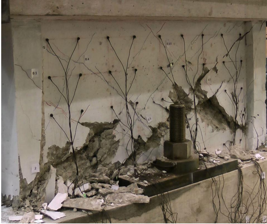
Figure 2-21 Failure (cracks width not measured) [15].
