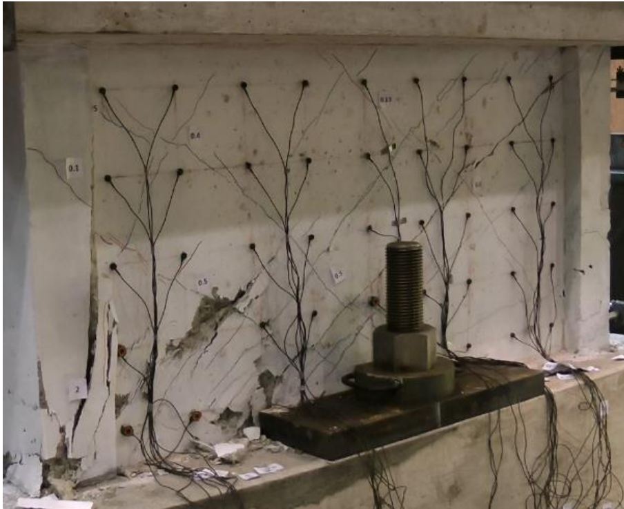
Figure 2-19 Failure (cracks width not measured) [15].
